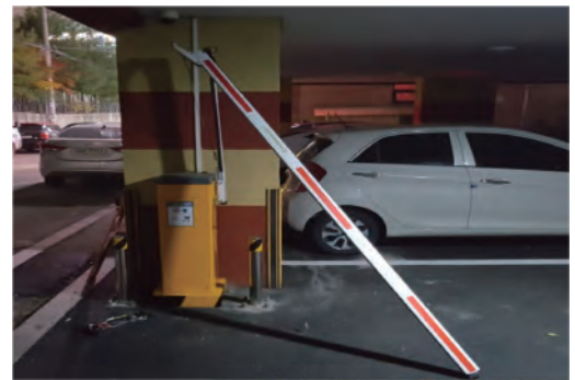
▲ Damaged or destroyed crossing gate
